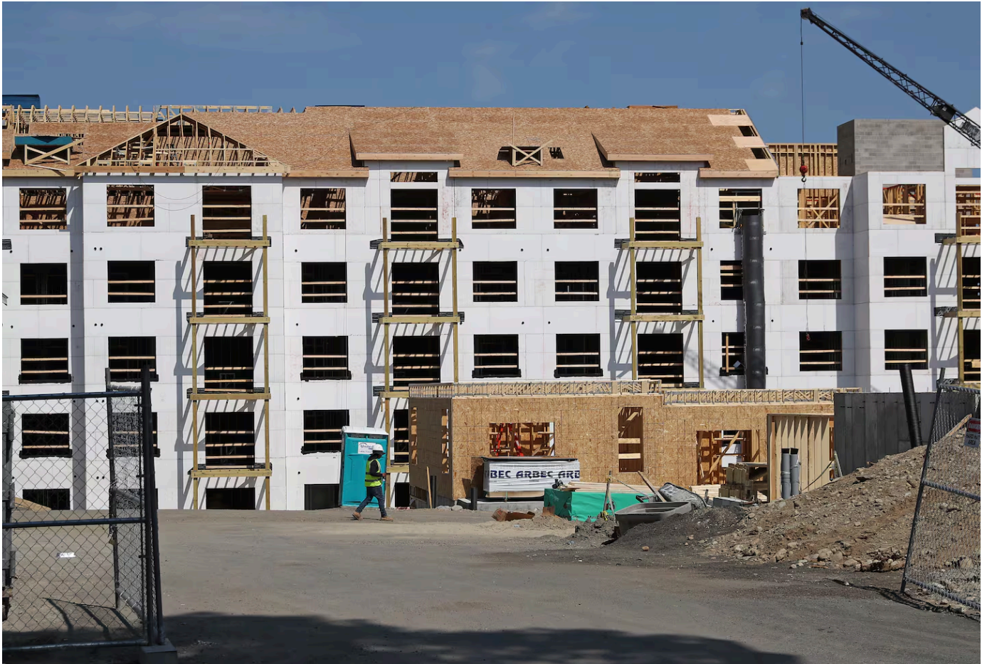
An apartment building under construction in Needham in 2017. DAVID L. RYAN/GLOBE STAFF FILE
